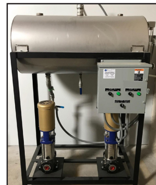
Boiler Feed Systems
